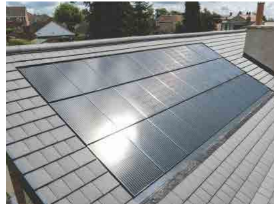
*PV laid against a slate roof.
