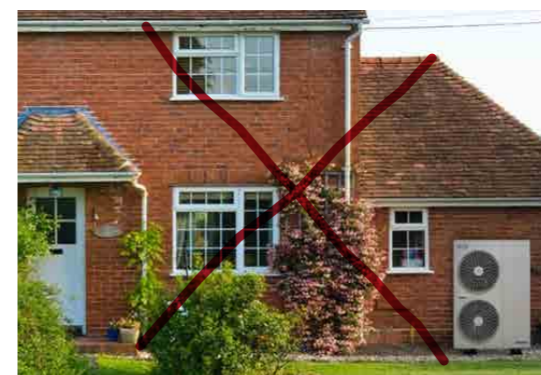
An ASHP on the front of a building.
