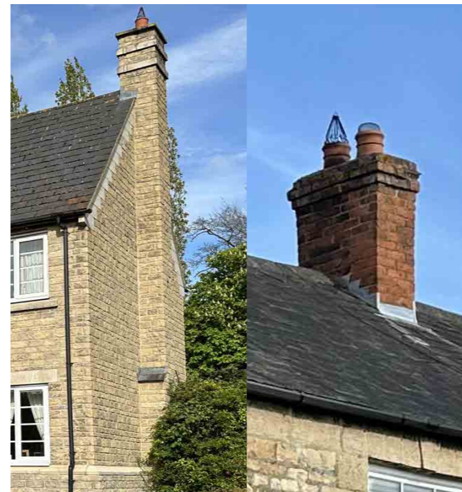
Example of existing gable end masonry and mid-roof chimney in Great Oakley Village.
