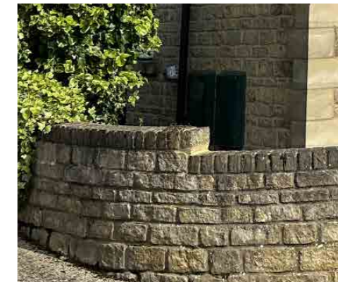
Meter box on a side wall.
