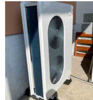
ASHP on the rear of a building.
